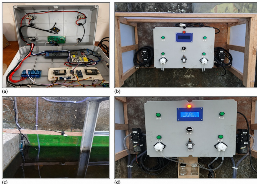
Figure 6. Physical Integration and Field Deployment of the HidroPond IoT System: (a) Integrated Control Panel, (b) Actuator Installation, (c) Sensor Installation, and (d) Operational Field Deployment.
